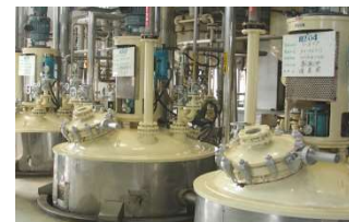
3,000 L Glass Lined Reactors
